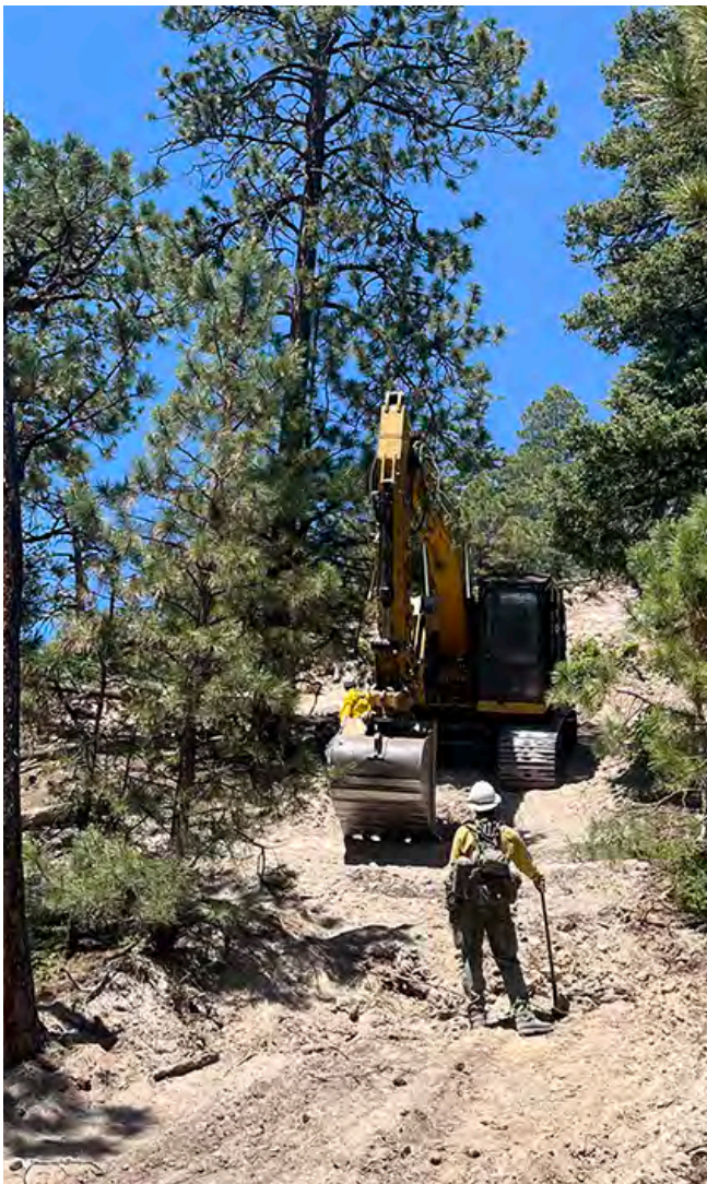
An excavator is used to rehabilitate firelines and roads following the Indios Fire. Credit/ Marija Osipchuk/BLM
