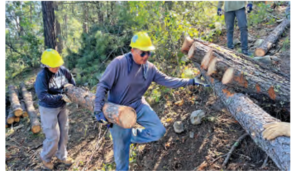
Forest Stewards Youth Corps crews build "trash racks" to slow water, debris, and prevent erosion in sensitive landscapes.
